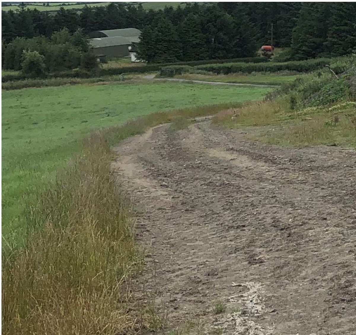
Photo 15-19: Spoil and bare ground
